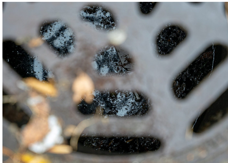
Sanchez says the storm drain down his block in Cicero frequently gets clogged and overflows after just a few days of light rain. Efrain Soriano for Borderless Magazine
