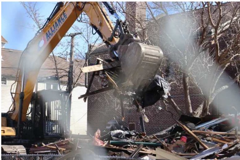
An excavator moves pieces of an abandoned Roseland house at 160 E. 111th Street on March 28, 2022. Credit: Maia McDonald/Block Club Chicago
