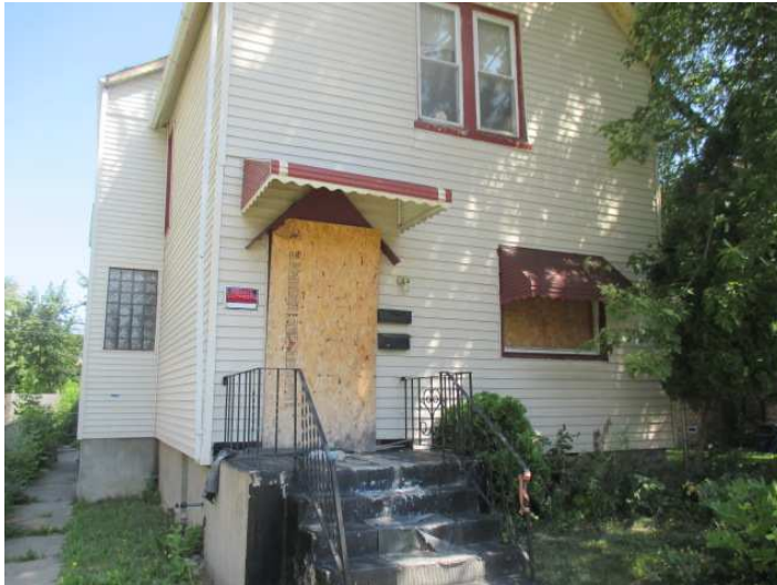
The house at 160 E. 111th St. in Roseland before it's demolition on March 28, 2022. Credit: City of Chicago Vacant Buildings
