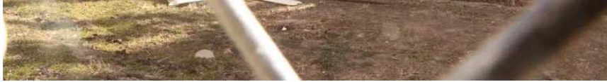
Crews demolish an abandoned house at 160 E. 111th Street where a community member was shot and killed the week before, on March 28, 2022.
