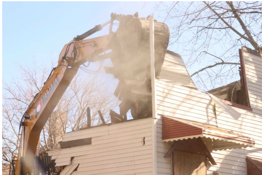
Crews demolish an abandoned Roseland home on March 28, 2022. Credit: Maia McDonald/Block Club Chicago
