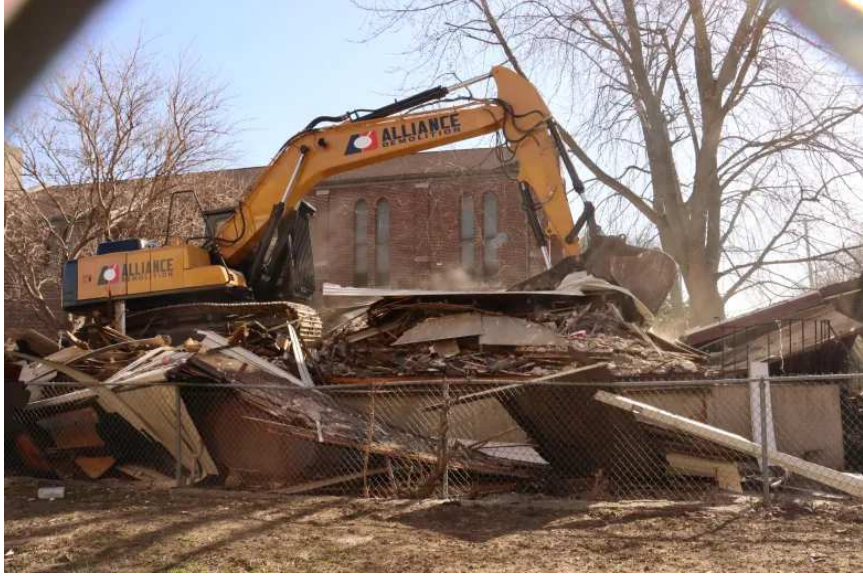
A crew demolishes an abandoned Roseland house at 160 E. 111th Street on March 28, 2022. Credit: Maia McDonald/Block Club Chicago
