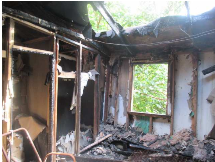
Fire damage at the house at 160 E. 111th St. before it's demolition on March 28, 2022. Credit: City of Chicago Vacant Buildings
