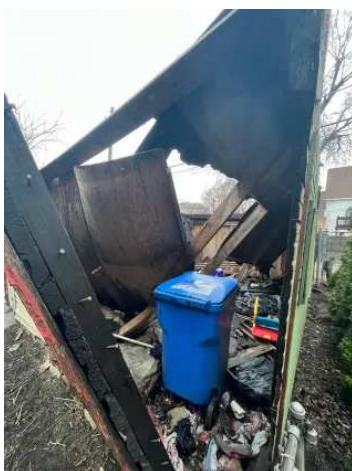
The collapsed garage at 160 E. 111th Street a week before its demolition on March 28, 2022. Credit: Arlene Echols
