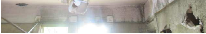
The roof of the house at 160 E. 111th St. before its demolition on March 28, 2022. Credit: City of Chicago Vacant Buildings
